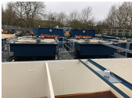
Figure 3 Containerised Temporary Plant Setup (stream A right, stream B left of photo)
