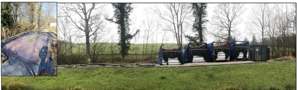
Figure 6 Passive Treatment Pilot Plant from right to left (Feed Tank; BCR1, 2, 3, 4; Reed bed (APW) 1, 2, discharge holding pond showing purple/white bacteria)
