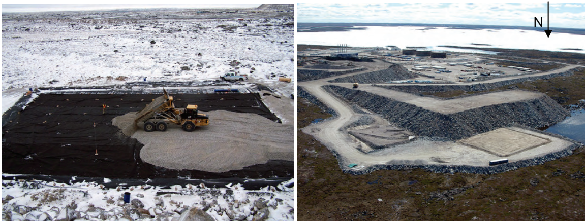
Figure 3. Photo to the left shows crushed rock being place over the impermeable liner of the Type I rock pad. Photo to the right shows the positions of the Type I pad (left) and Type III pad (right). The dimension of each pad is 50 m × 60 m. The L-shaped ramp adjacent to the test pads in the foreground will be used to tip rock onto the pads for construction of the waste rock piles. The arrow to the right of the photo is pointing North.
