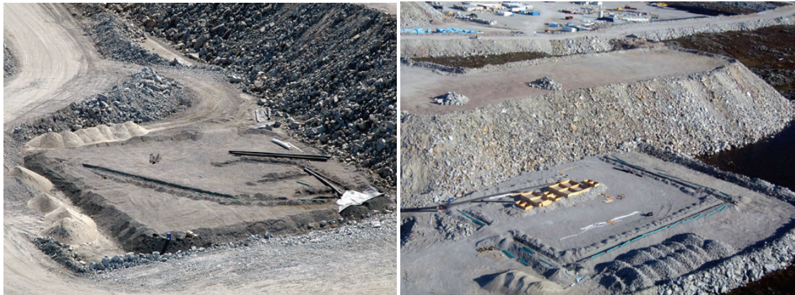
Figure 4. Photo to the left shows the basal drainage ditch excavated diagonally across the center of the Type I pad exiting through the SW corner. Photo to the right shows the basal drainage ditches excavated around the perimeter of the Type III pad exiting through the SW and NW corners.
