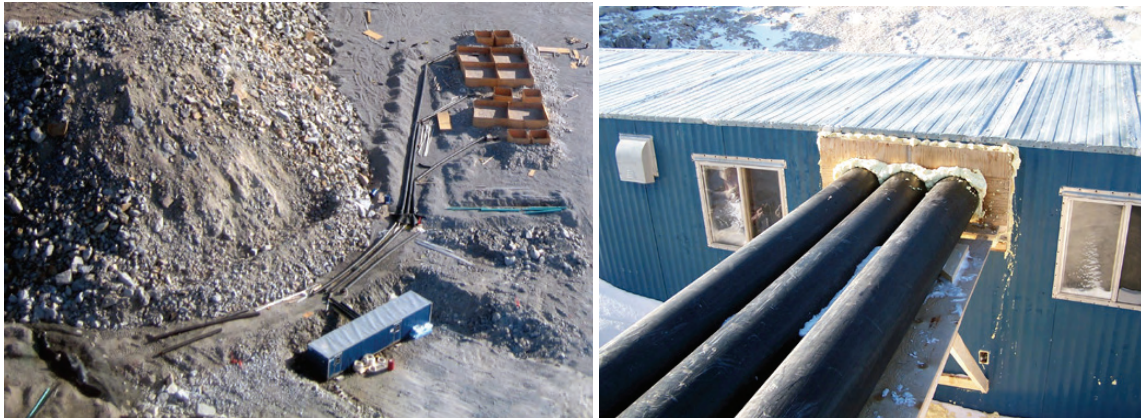
Figure 6. Photo to the left shows cluster lysimeter drainage pipes directed into the instrumentation shack. The instrumentation shack is situated between the Type I and Type III rock pads. The photo to the right shows lysimeter drainage pipes entering the instrumentation shack.
