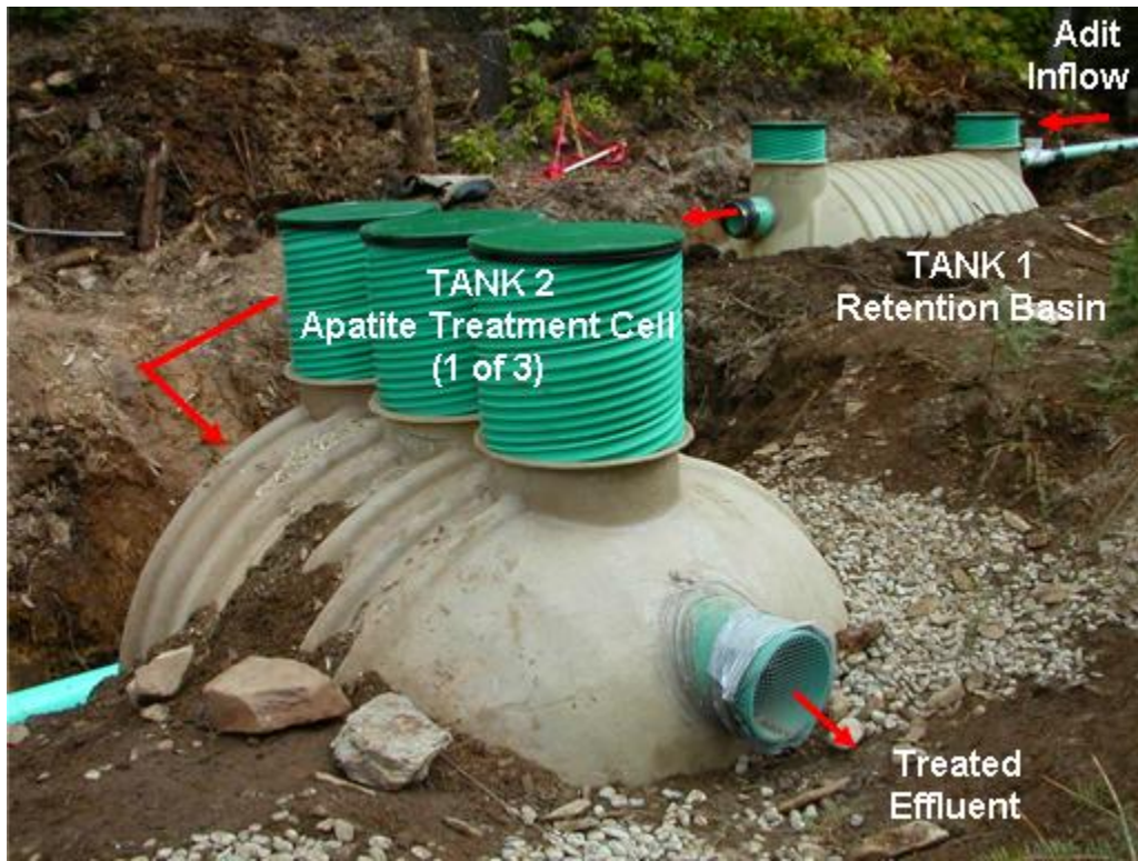
Figure 2. Photograph of the Treatment System During Construction (white treatment tanks with green manholes for access).
