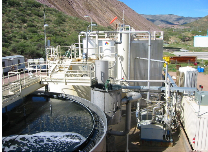
Figure 5. BioSulphide® Plant for copper recovery at Bisbee, Arizona
