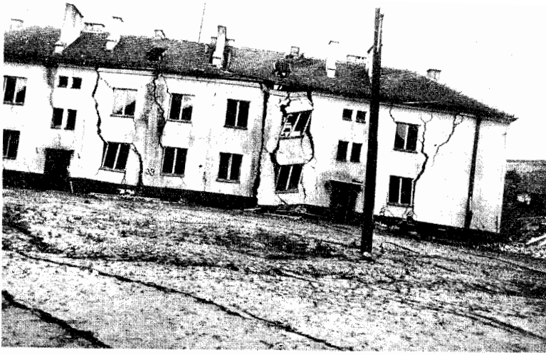
Fig. 9 Photography of damaged building
